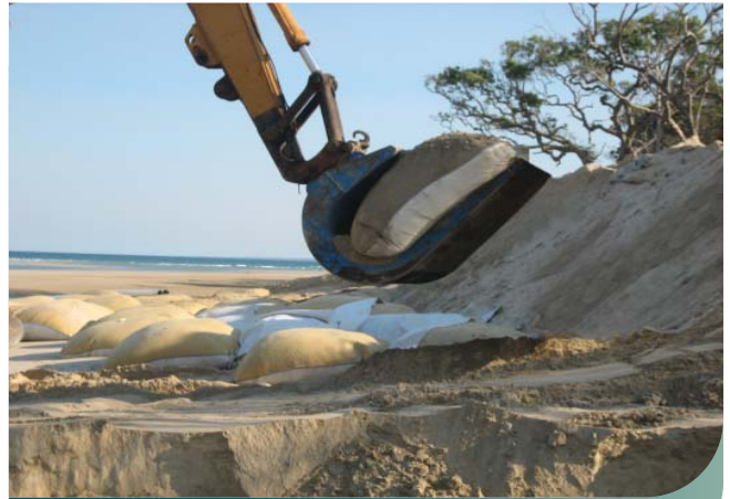
Figure 14. Sand container placement
