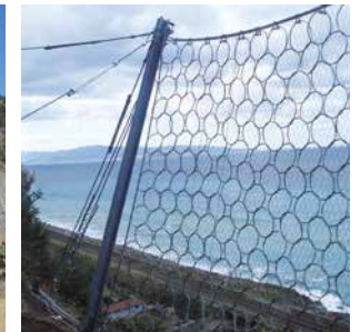
5 Dynamic Rockfall Barriers
