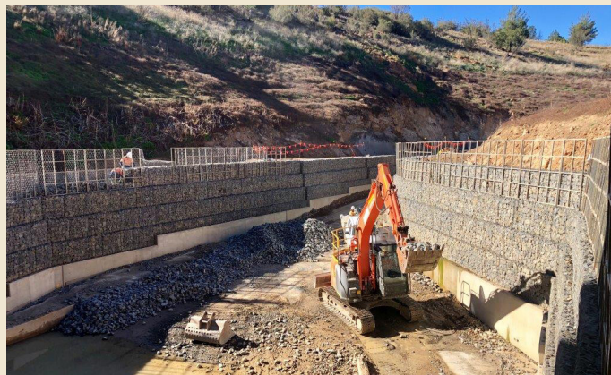
The structures have been installed to a very high standard and have received several commendations.
