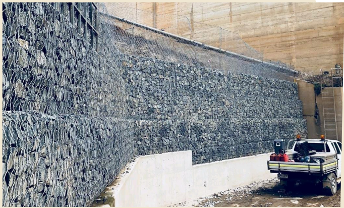
The Terramesh system was selected due to the reduced rock quantity required and relatively narrow width due to the existing rock slope.
