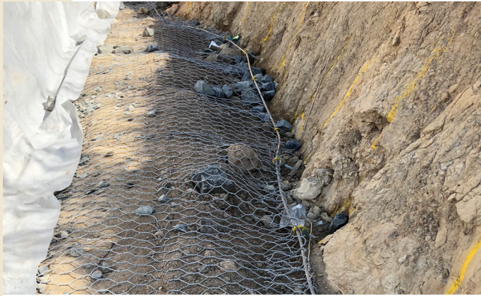
Anchors to secure the Terramesh soil reinforcement to the rock face due to space constraints.
