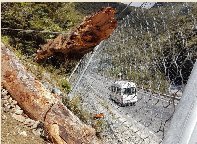
Fallen trees stopped from falling onto the road by the fence.
