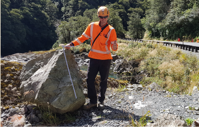
Recorded historical data shows that rockfalls at this site are between 0.2 m and 1 m in diameter.
