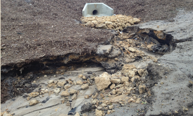
Outlet erosion before the solution
