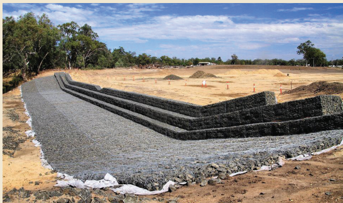
The install only took five weeks out of the allowed eight weeks
