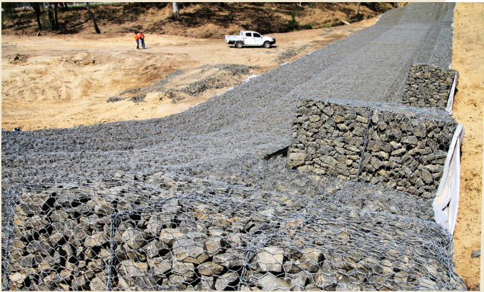
In total 572 m 3 of Gabions over three sizes and 4008 m 2 of 230 mm deep Reno Mattresses were installed
